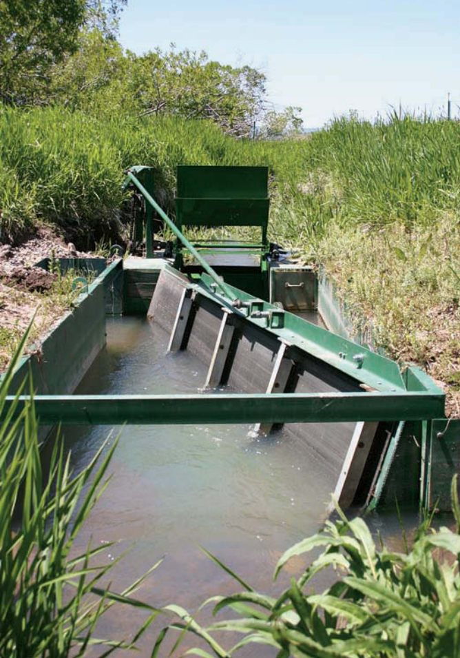
A self-cleaning fish screen at a stream-flow diversion on lower Lassen Creek prevents fish from entering irrigation delivery ditches and becoming stranded.
