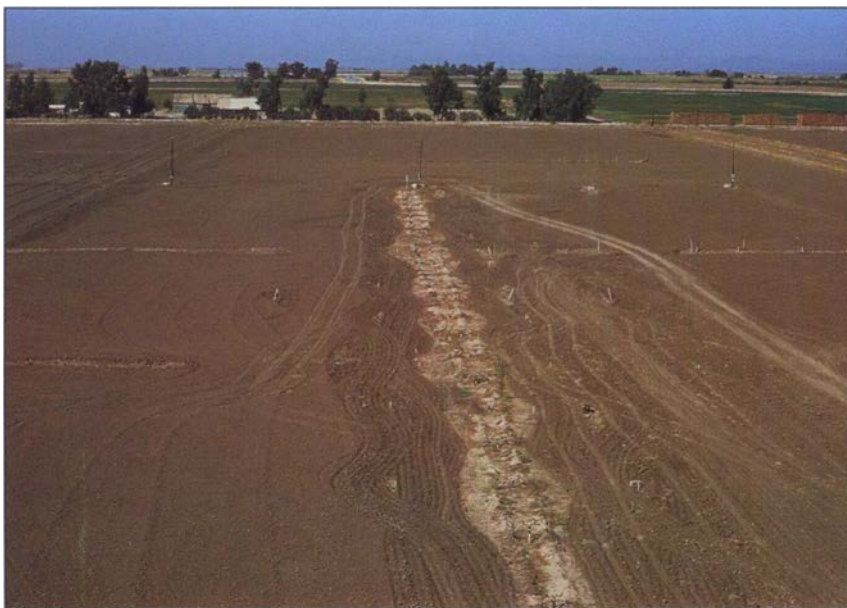
In an effort to control salinity associated with a shallow artesian aquifer, a shallow “skimming” drainage well system was installed.
