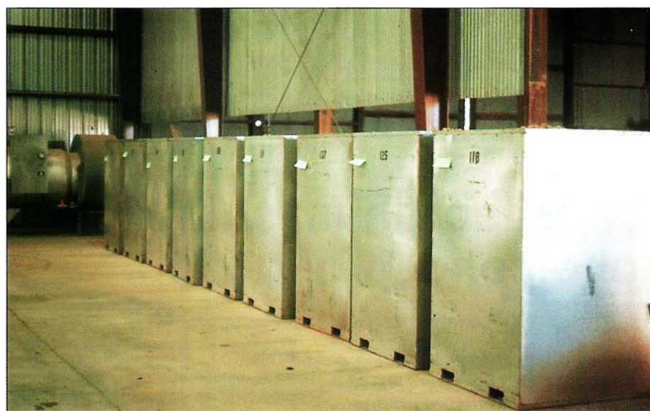
In a pot-hole dehydrator, heated air enters through the bottom of the bins via an underground air tunnel from the burner.
