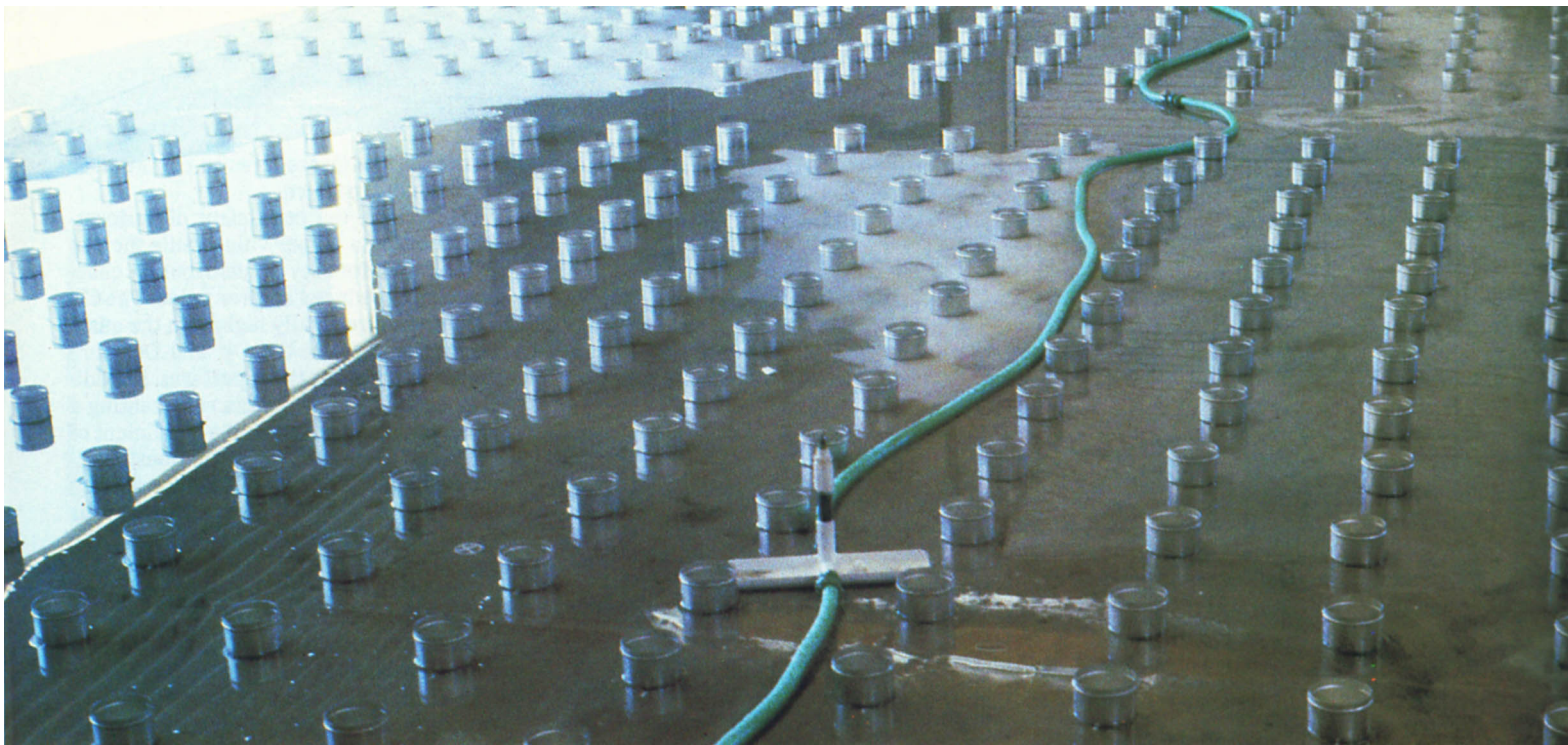
Catch cans laid out in a large warehouse to measure uniformity of low-flow sprinkler systems.
