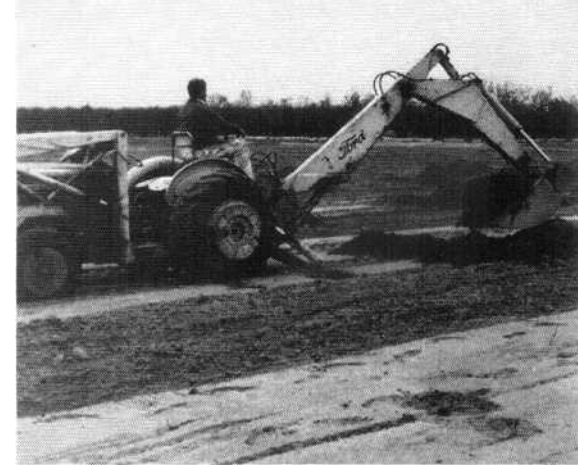
Tractor-mounted backhoe seen above was used in making excavations for tree planting and analysis of soil compaction and water penetration in this orchard study.
