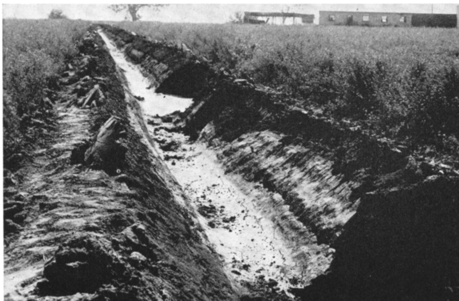
Collapse of a ditch section during irrigation.
