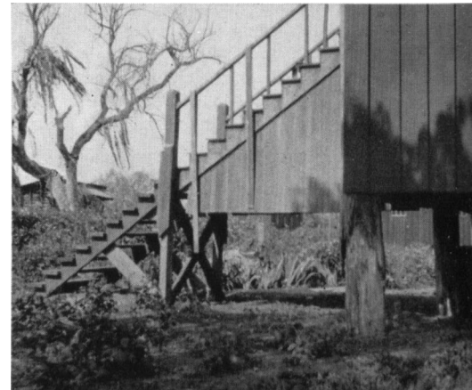
Buildings on pilings do not settle as the soil subsides. Note added steps.
