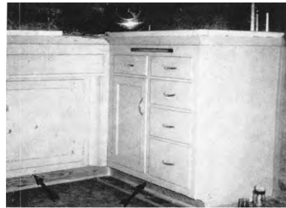
Kitchen cabinets with holes (indicated by arrows) drilled into kick panels for application of silica aerogel in the voids under these cabinets. Food and water containers may be seen at the lower right-hand corner of the figure.
